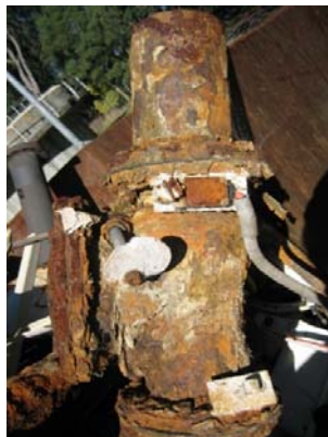
Photograph 1: An example of corroded equipment at a WWTP (Photo: Alan Neethling)
