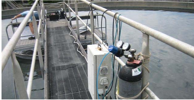
Photograph 2: A sensor package was deployed from the gantry into the primary clarifier tank. The housing for a power supply is visible in the foreground. A second sensor was installed at the plant inlet. (Photo: Alan Neethling)
