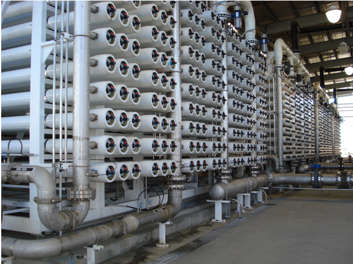
Photograph 5: Reverse Osmosis System
