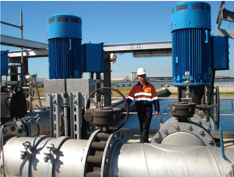
Photograph 1: Raw water pumps (clarifier feed)
