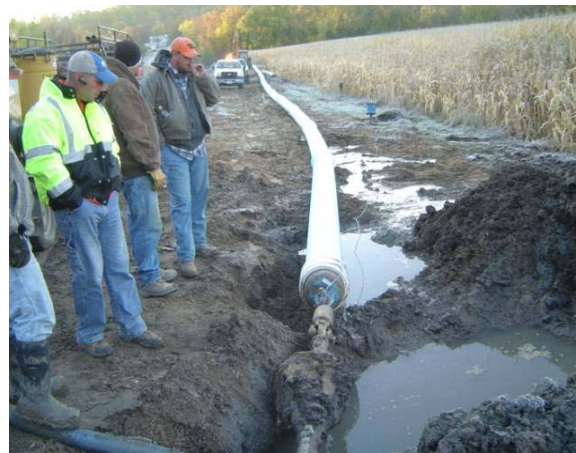
This project in central Iowa shows how quick-and-easy internally restrained PVC pressure pipe can be installed by HDD.
