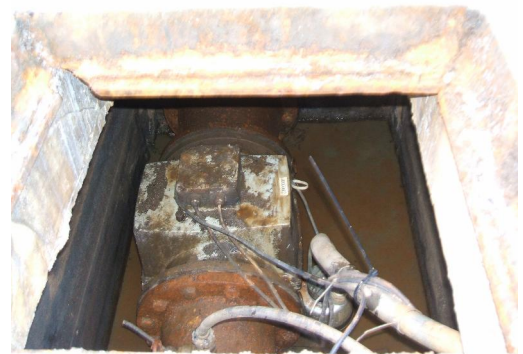
Figure 12 Typical CCC Flowmeter in chamber
