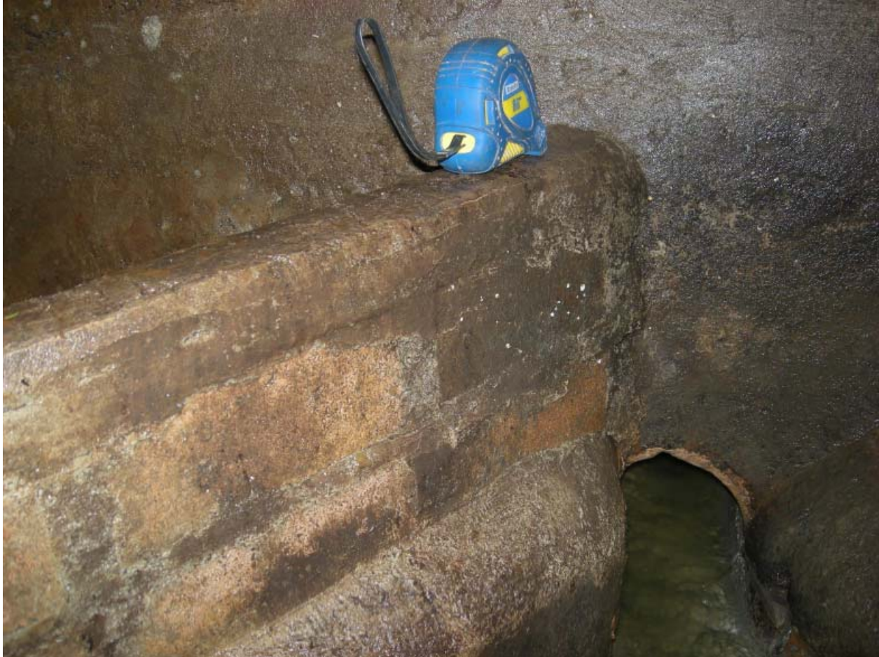
Photograph 1: Photo from Field Inspection Contractor when Requested to Include Tape Measure on Weir
