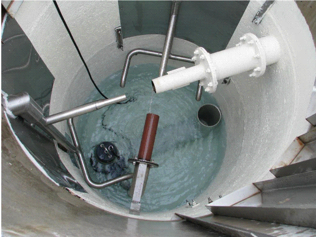
Photograph 1: Aeration chamber pipe work arrangement
