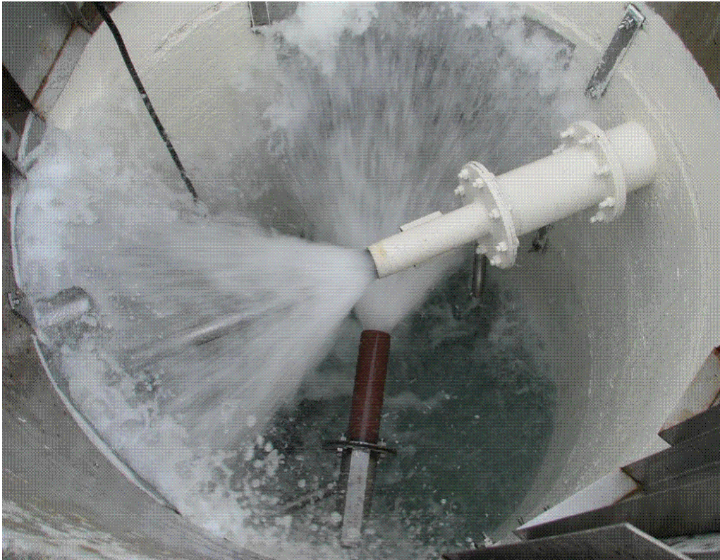
Photograph 2: Vortex Accelerators operating
