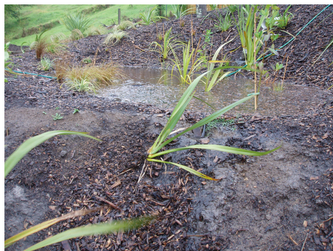
Figure 8: Overflow bank erosion at Kia Ora Road rain garden, Birkenhead
