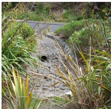
Figure 5: Inlet channelization protection (Rangitoto College site, Northshore)
