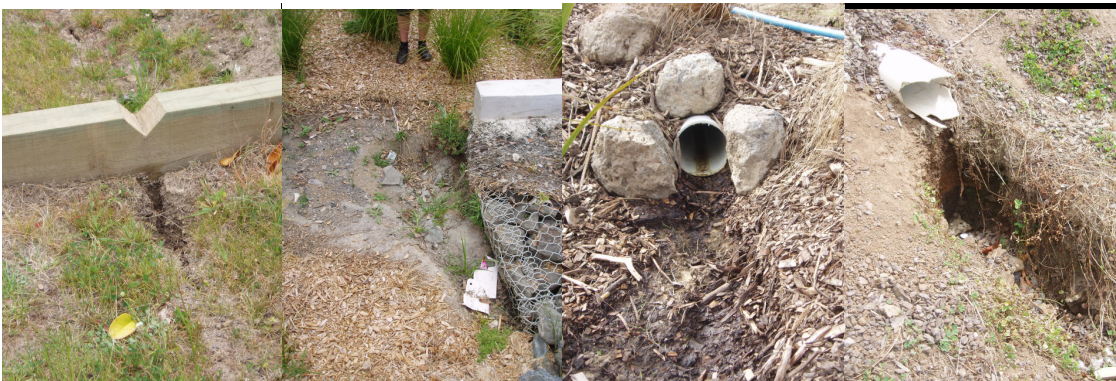
Figure 4: Inlet erosion at St Lukes, Karaka Cove, Kia Ora and Oranga Community centre rain gardens
