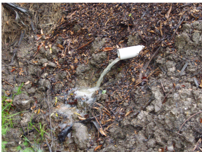
Figure 7: Outlet erosion at Kia Ora Road rain garden, Birkenhead
