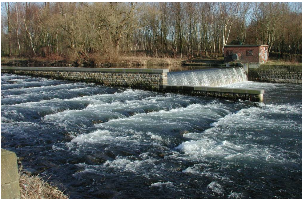
Photograph 5: Rock-ramp fishway entrance parallel to the river flow at the Reuschenberger Mühle Weir, Wupper River, Germany
