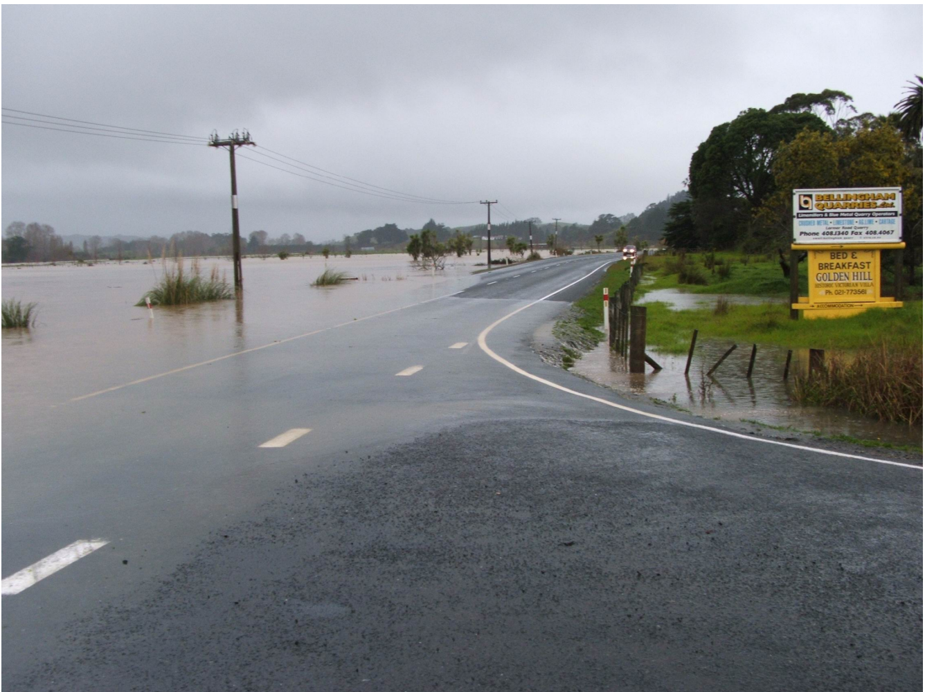
Figure 4: Photographs Indicating Flooding of SH1 during July 2007 Storm Event
