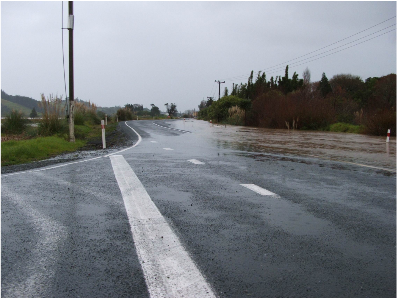
Figure 5: Photographs Indicating Flooding of SH1 during July 2007 Storm Event
