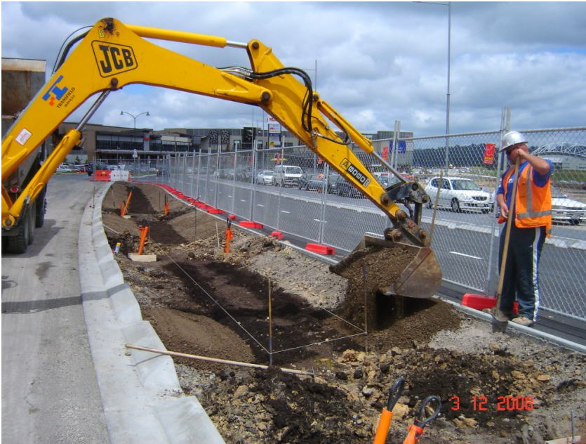
Photo 3: Median raingarden during construction showing tree pits, continuous medium trench and sideslope soil
