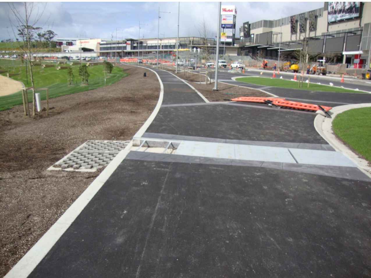
Photograph 6: Bioretention swale with tree pits between paths. Grassed areas on right. Footpath channel discharging to swale and bioretention trees pits foreground and left.
