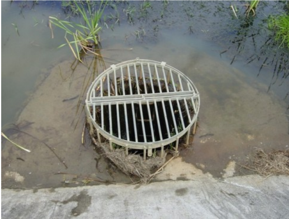
Figure 8: Outlet (debris screen) before restoration
