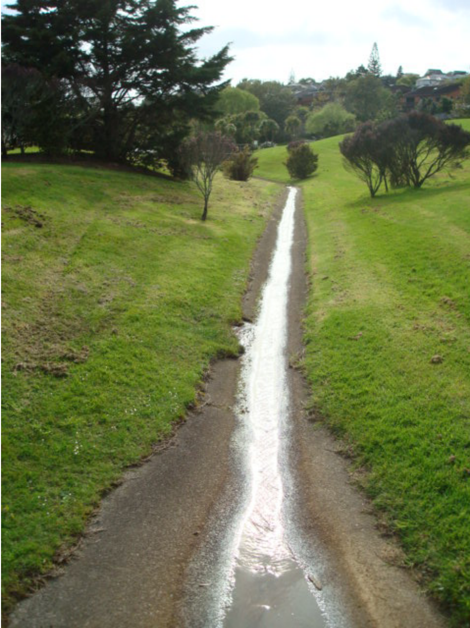
Figure 5: Northern concrete channel before restoration
