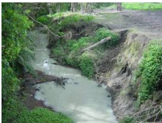
Figure 2: Stream bank erosion infestation
