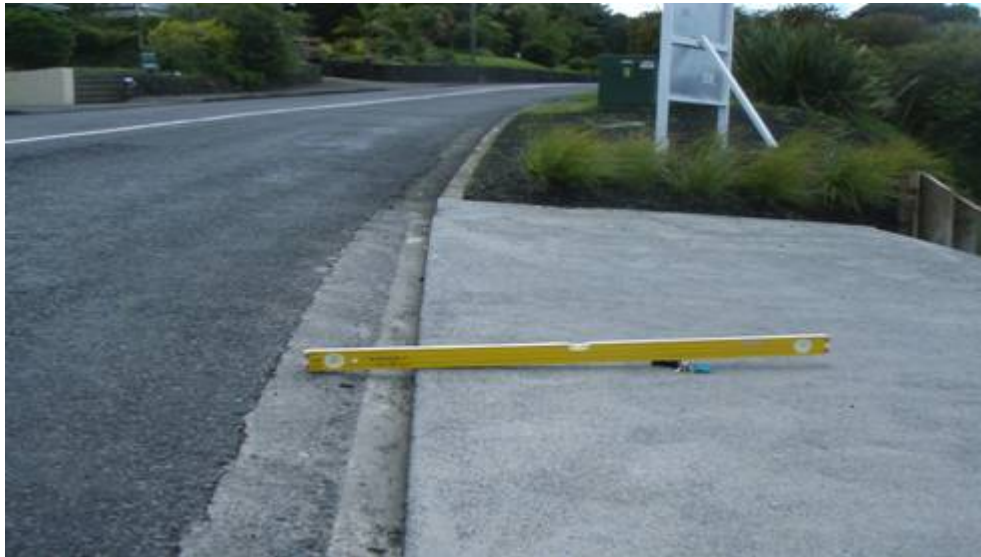
Photograph 1: Vehicle Crossing Installed By the Developer Without Roll-Over To Retain Flow In Road Channel. Channel Flow Estimated To Be 0.2m 3 /sec In A 50% AEP Storm
