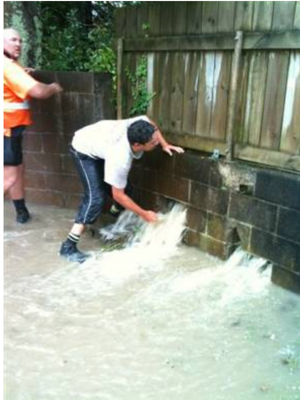
Photograph 4: Breaking Restrictive Fence to Allow Overland Flow Through (Action Taken Too Late In This Case)
