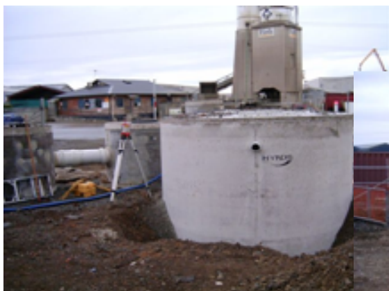
Figure 7: All units partially buried (looking at the water storage tank)
