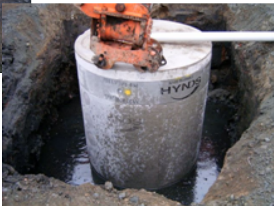
Figure 6: Upstream pump chamber (IMH-A)
