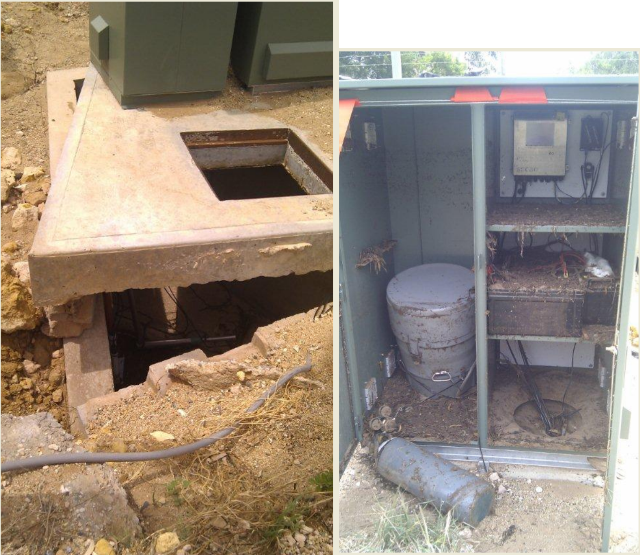
Image 15: Destruction after Flood
