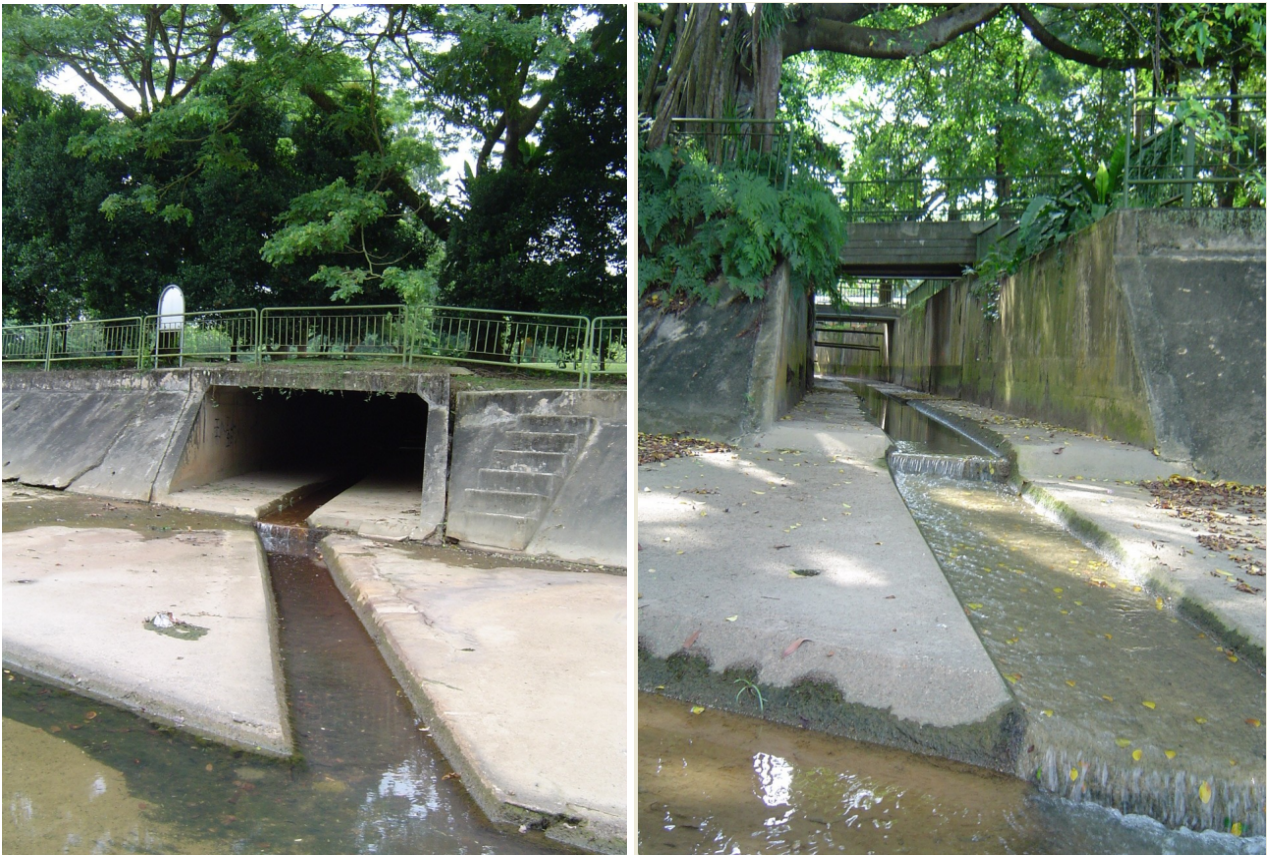
Image 3: Typical drain structures
