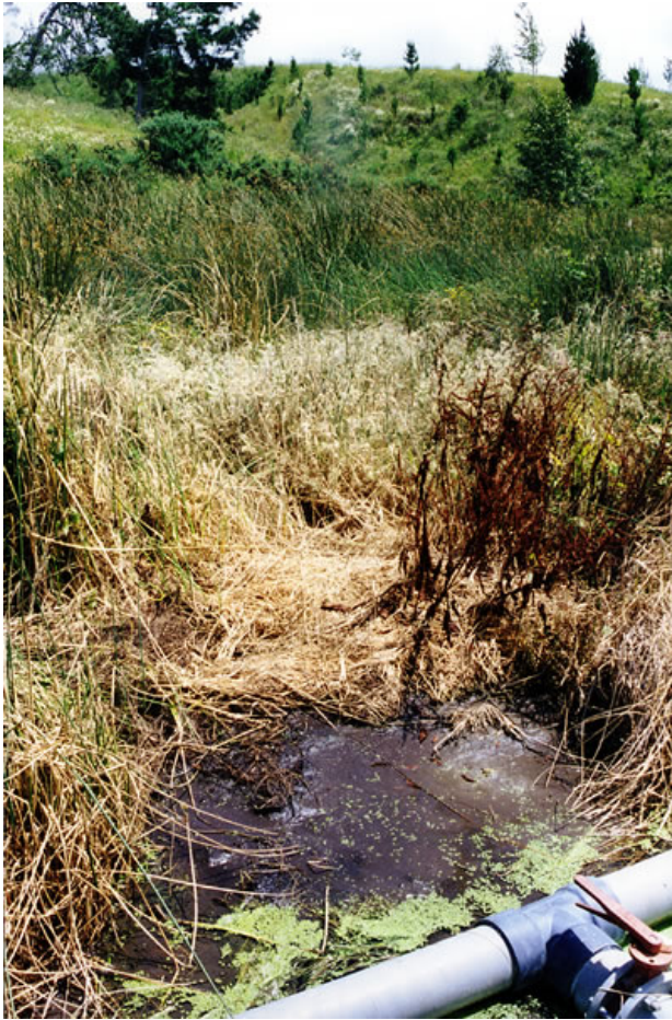
Photo 2. It is important to avoid excessive sludge carry-over into constructed wetlands from preceding treatment stages. Sludge accumulations can promote weed invasion and affect the treatment performance and operational lifetime of constructed wetlands.
