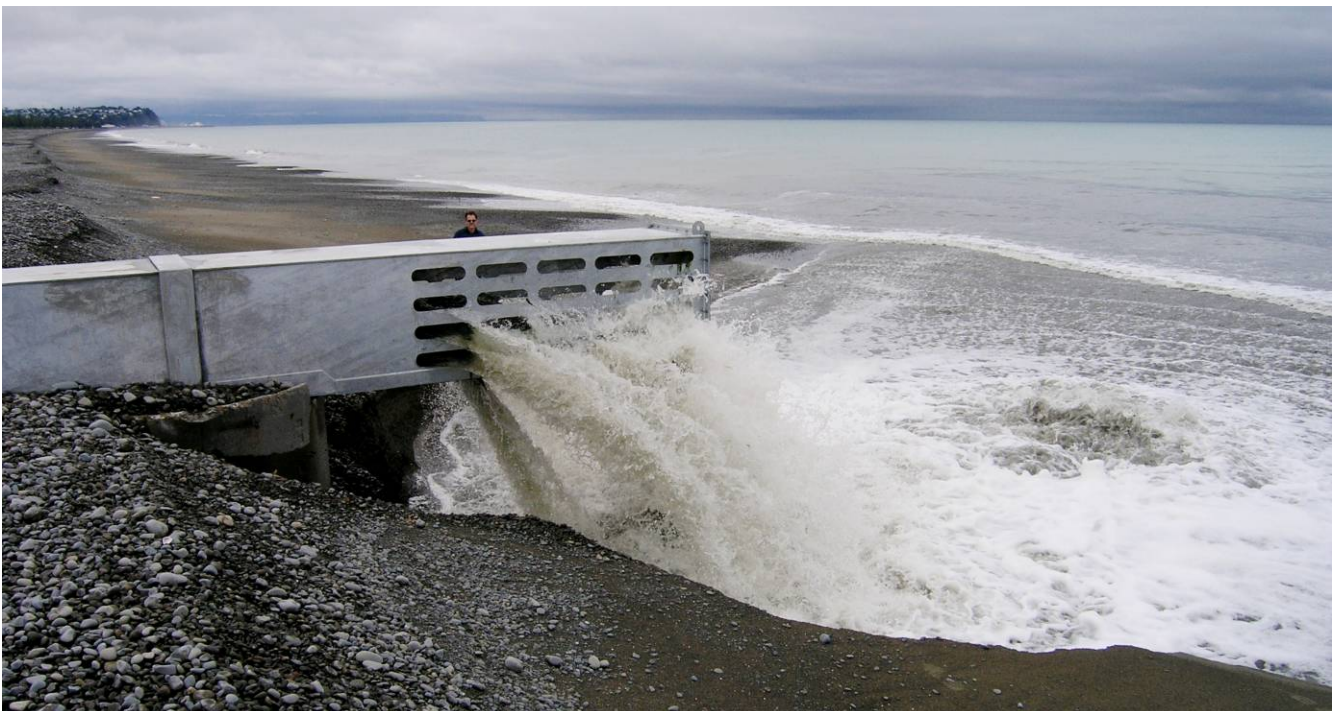
Photograph 5: Service pump and drainage outlet
