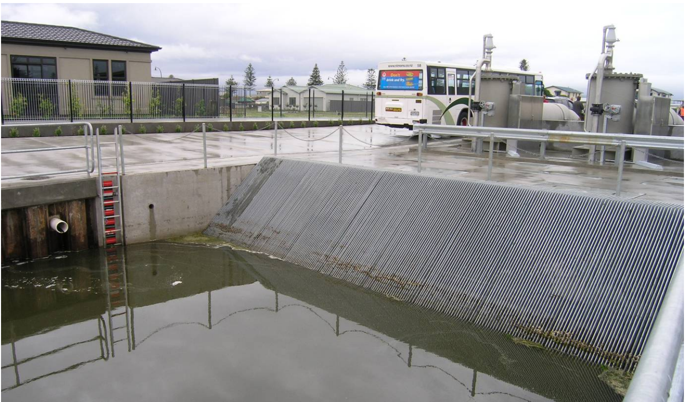
Photograph 2: Pump station intake screens and pumps
