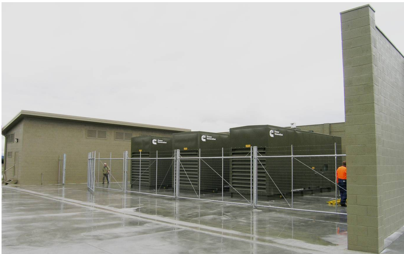
Photograph 3: Diesel generators and noise wall (viewed from golf course side), with control building at left rear
