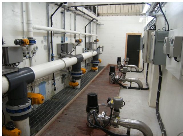
Photograph 7: Upgraded filter gallery
