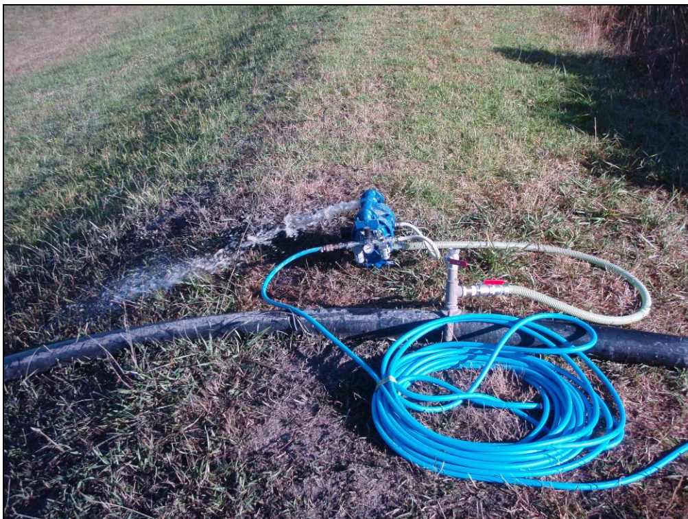
Photograph 3: Siphon Priming System.
