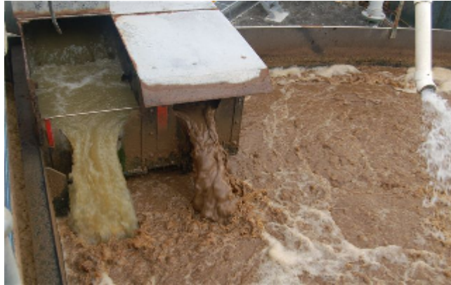
Figure 3: Raw sewage inlet to SBR
