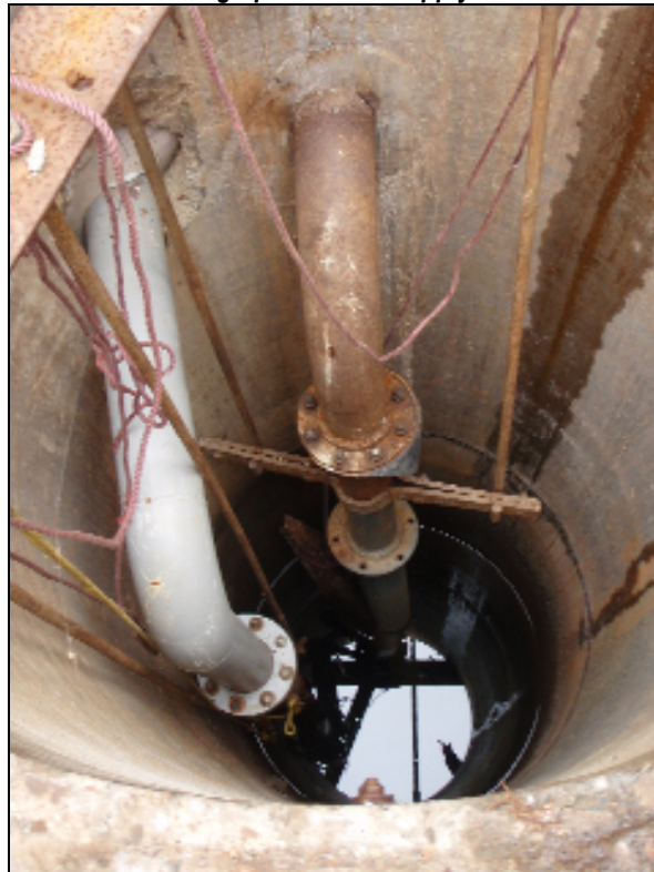
Photograph 1: Water supply well
