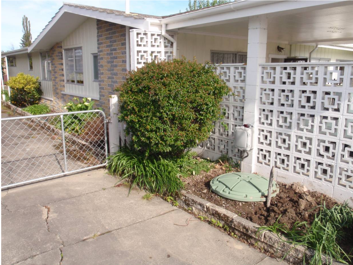
Photograph 4: Installed Grinder Unit and Control Panel
