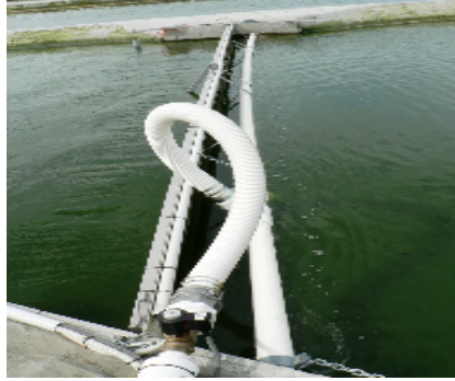
Figure 5: Photograph of the Christchurch Demonstration HRAP CO 2 addition sump
