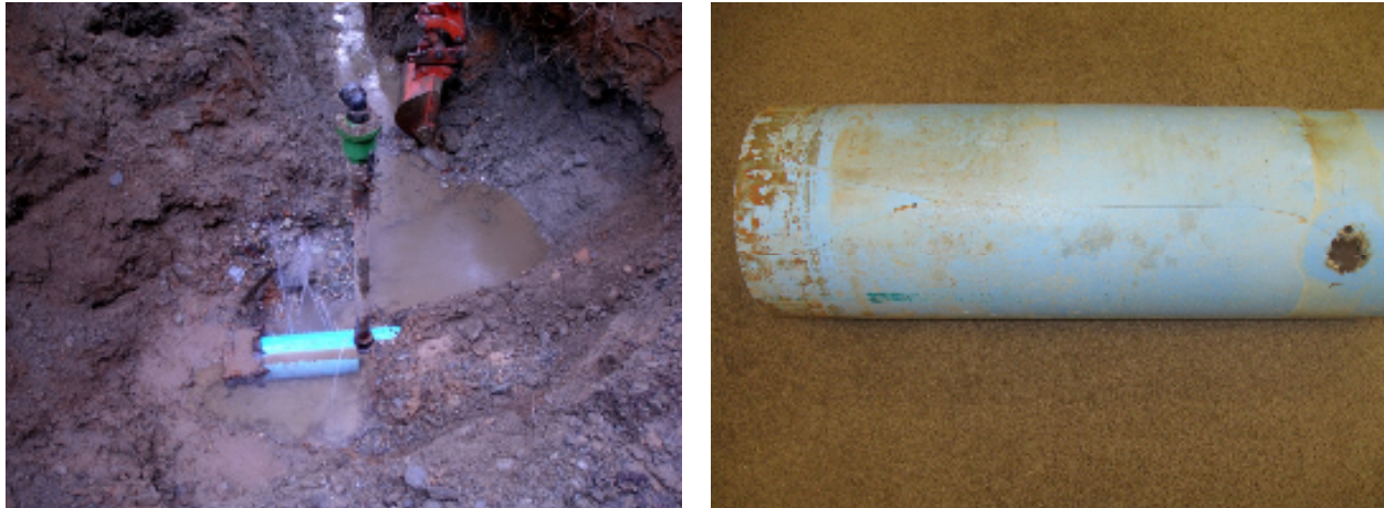
Figure 6: Section of broken pipe from 3rd burst (a) in-situ, (b) showing method of drilling tapping point
