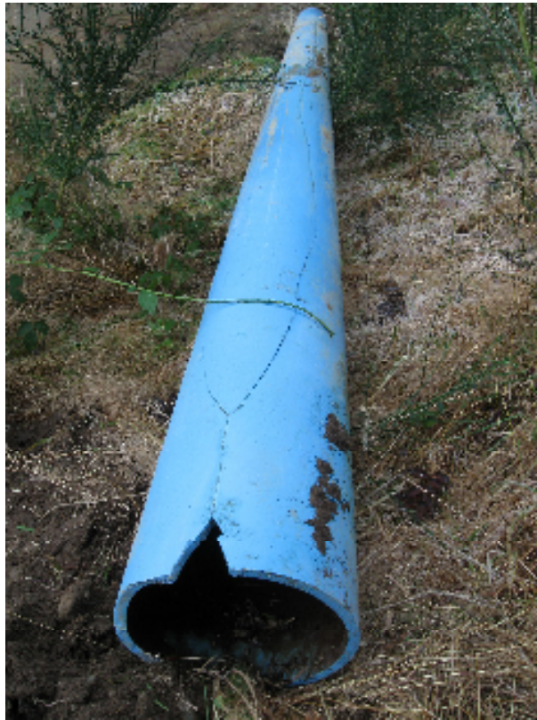
Figure 3: Section of damaged pipe, 1st burst
