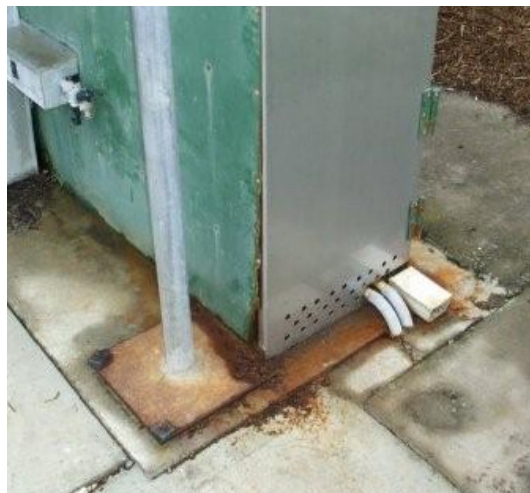
Photograph 2: Corrosion of control cabinet
