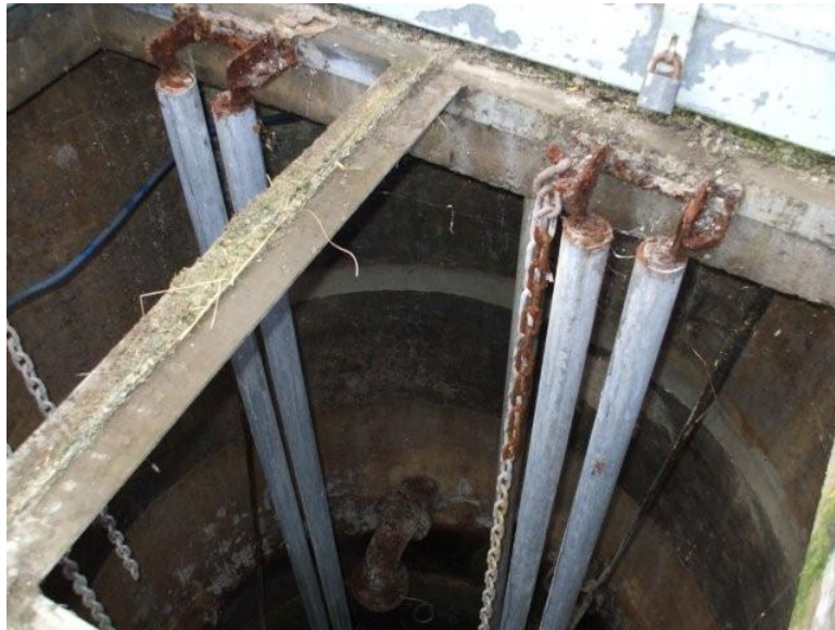
Photograph 1: Corrosion of wet well pump lifting chains and guide rail supports
