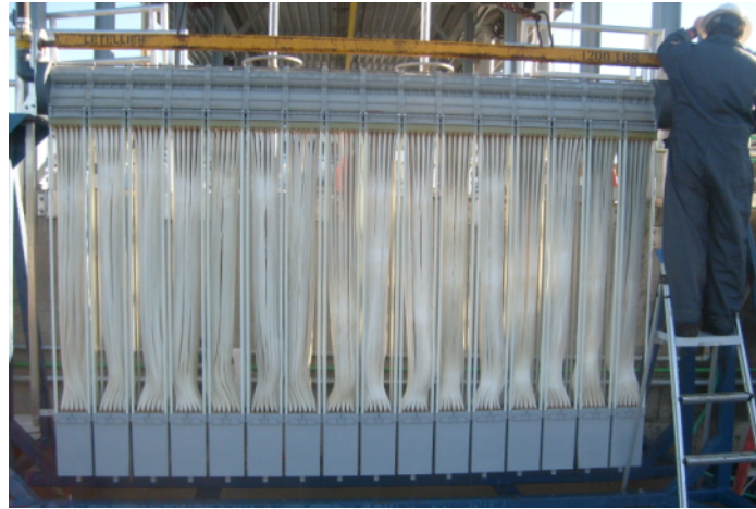
Photograph 1: Rack of MBR Membranes with pulsed flow device below each module
