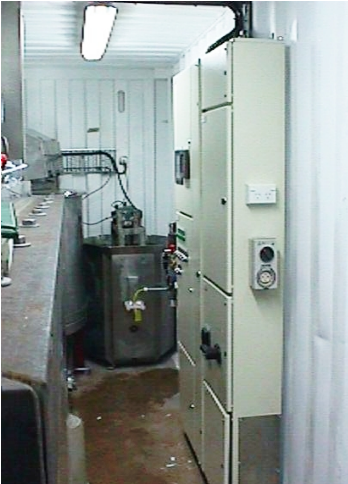
Photograph 3: Electrical section of Philippines containerised pilot plant – Reactors and powered ventilation to the left
