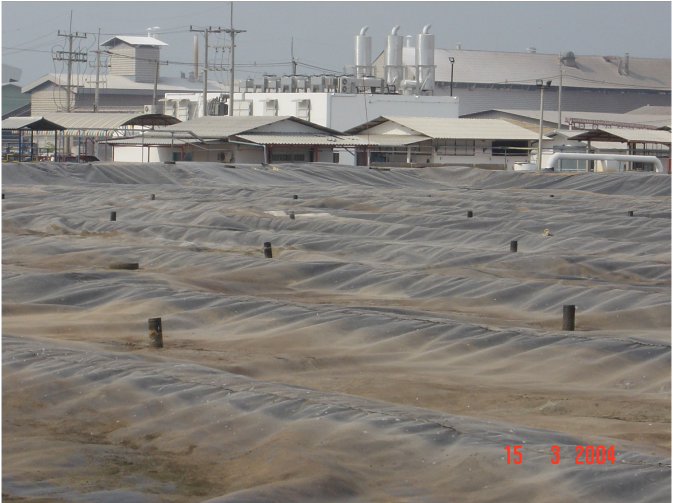
Photograph 1: The Khorat waste to energy plant looking across the CIGAR flexible gas retaining cover. The plant control is in the buildings just beyond the cover to the left. The three 1.3 MW generator exhaust silencers can be seen on top of the square generator building. The rear-most, tall building is part of the factory being supplied the biogas for its boilers approx 0.8 Km away
