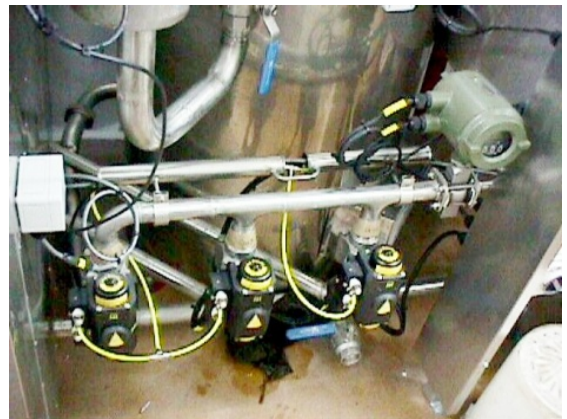
Photograph 4: Flow meter on right saved from attack by good sealing and cable glands
