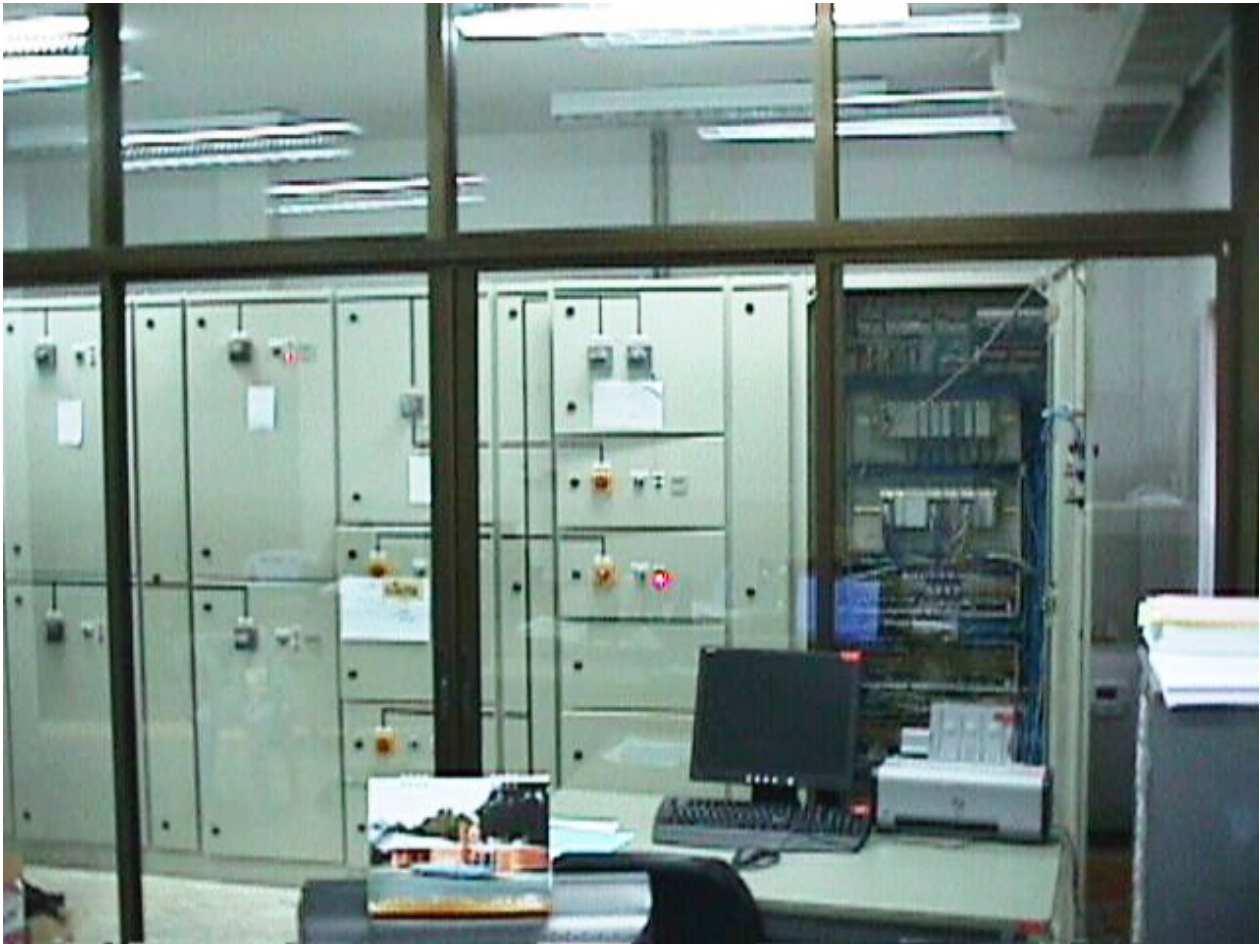
Photograph 7: Switchboard behind glass to allow observation with minimal need for personnel entry to reduce air exchanges
