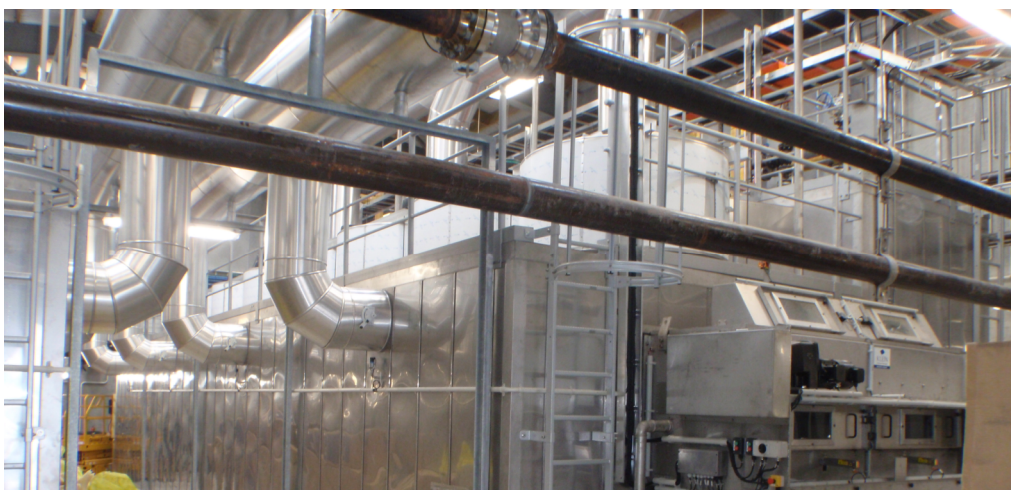
Photograph 2: Christchurch Biosolids Dryer Line 2
