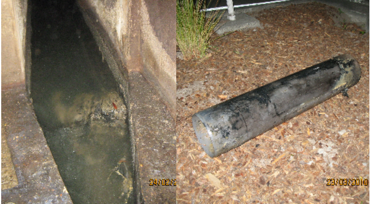
Photographs 1&2: Blocked Flume (AWT 3:35am), Obstruction Removed
