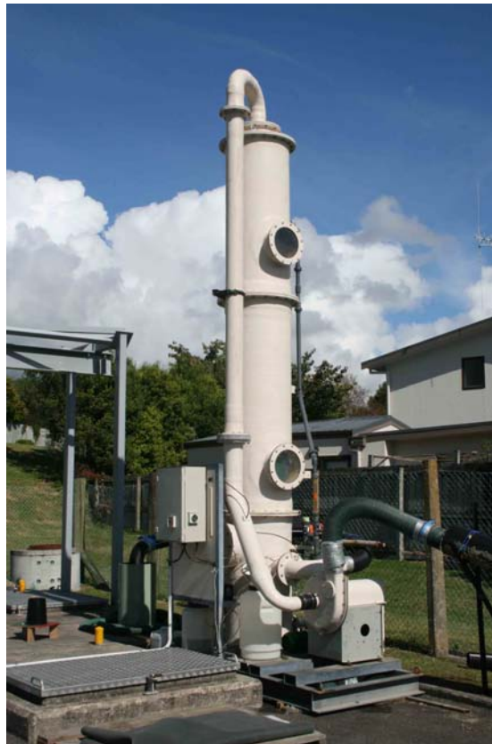
Photo 3: Biological Scrubber Trial at Otumanga Pump Station, Tauranga
