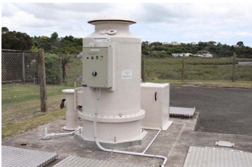
Photo 4: Otumanga Pump Station: Carbon adsorption bed with inlet filter, fan & acoustic housing
