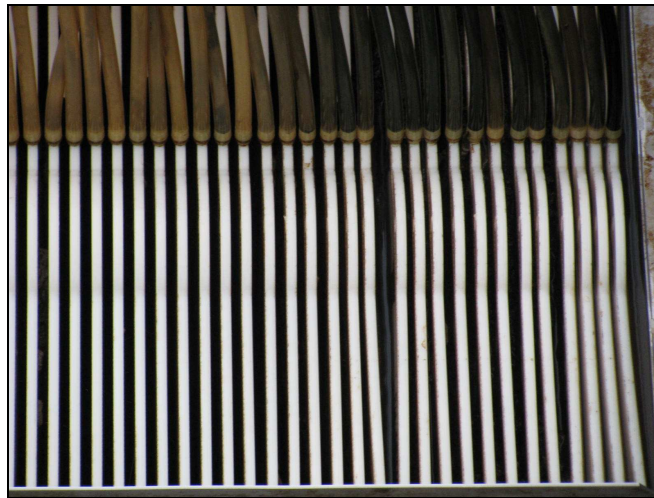
Photograph 2: Examples of severe sludge caking [from left; Te Aroha WWTP (26052010), Te Aroha WWTP (27052010)]
