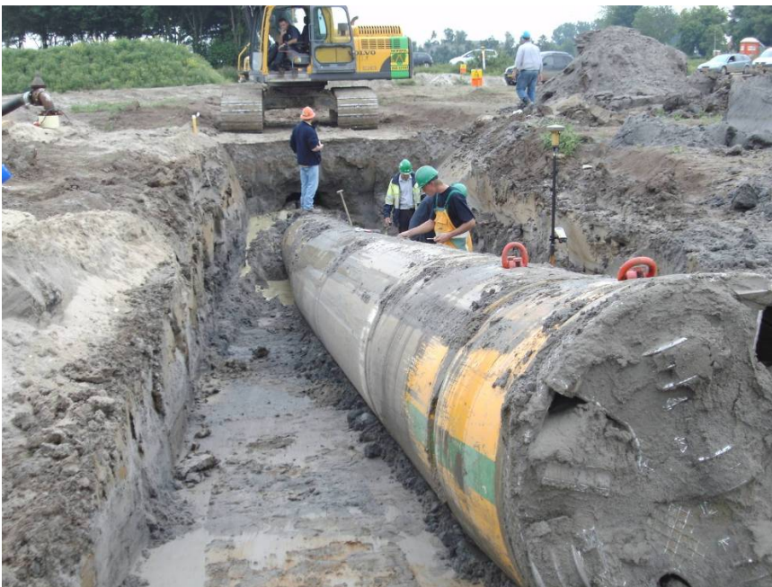
Figure 14: Arrival of the Direct Pipe-machine on the target side in Elst, Netherlands.
