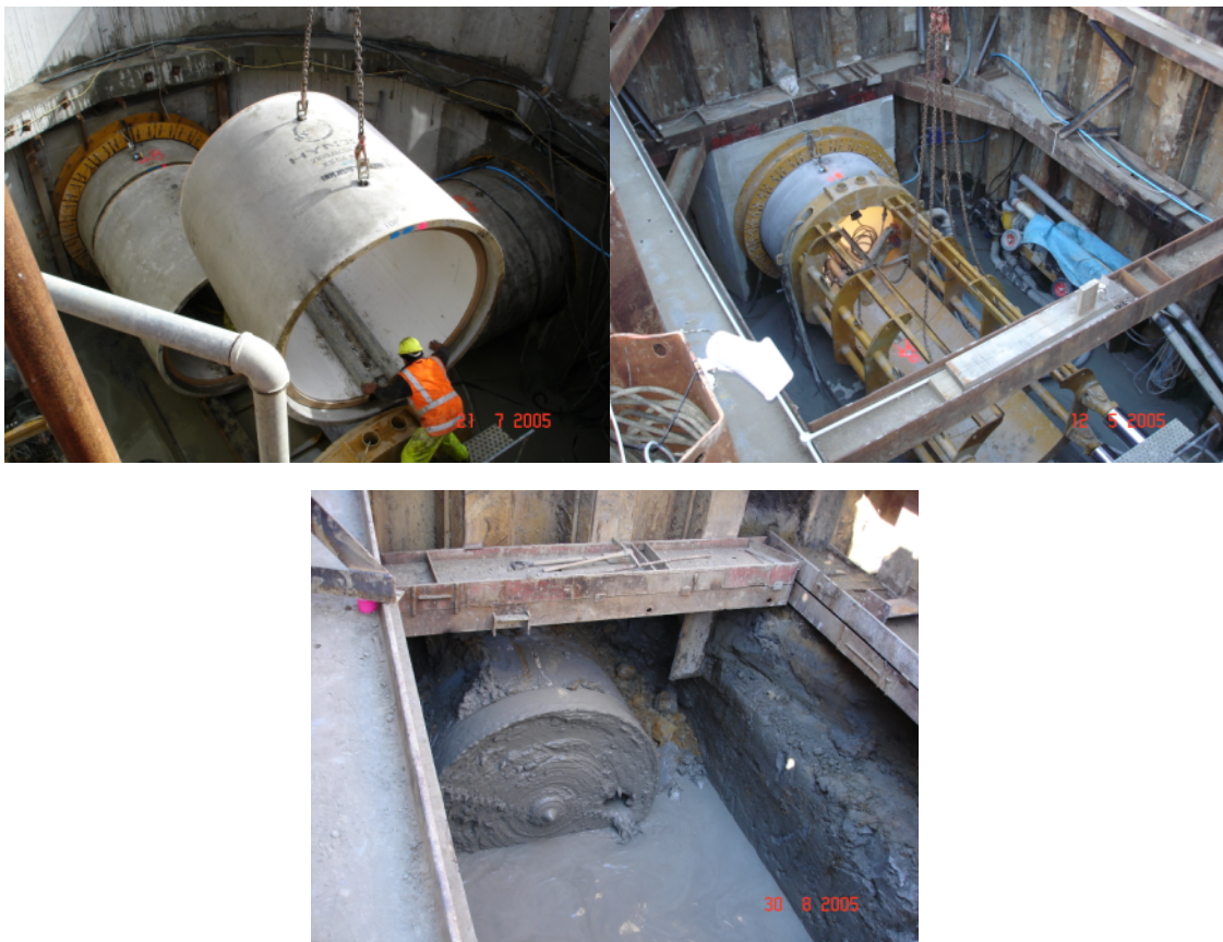
Photographs 1 to 3: Browns Bay 2.1m diameter pipeline - Installing Pipes Prior Jacking / Jacking Shaft / Micro tunneling Machine Head Entering Reception Shaft
