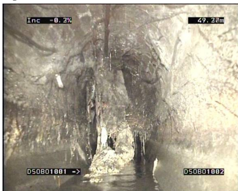
Figure 11 Root intrusions Branch 1
