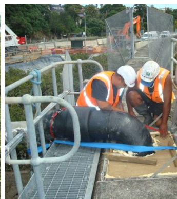
Figure 26 Bypass Pipe entry at Orakei Main
