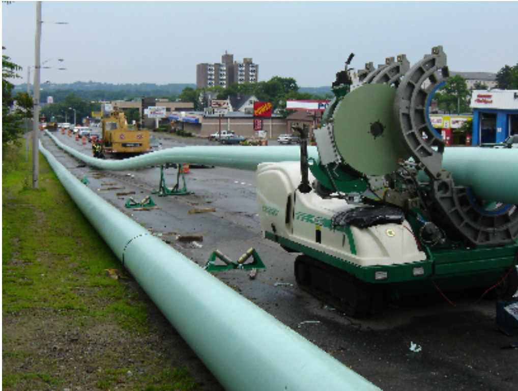
Photograph 3: Applying an intermediate weld between two FPVC™ welded strings for slip-lining of an existing concrete pressure sewer, USA.
