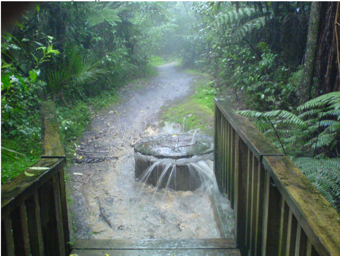
Picture 1: Overflowing manhole at Birkdale C
