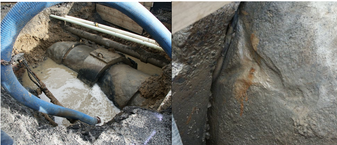
Photograph 3: General view of the leak site and close up of scoured pipe and dislodged rubber ring
