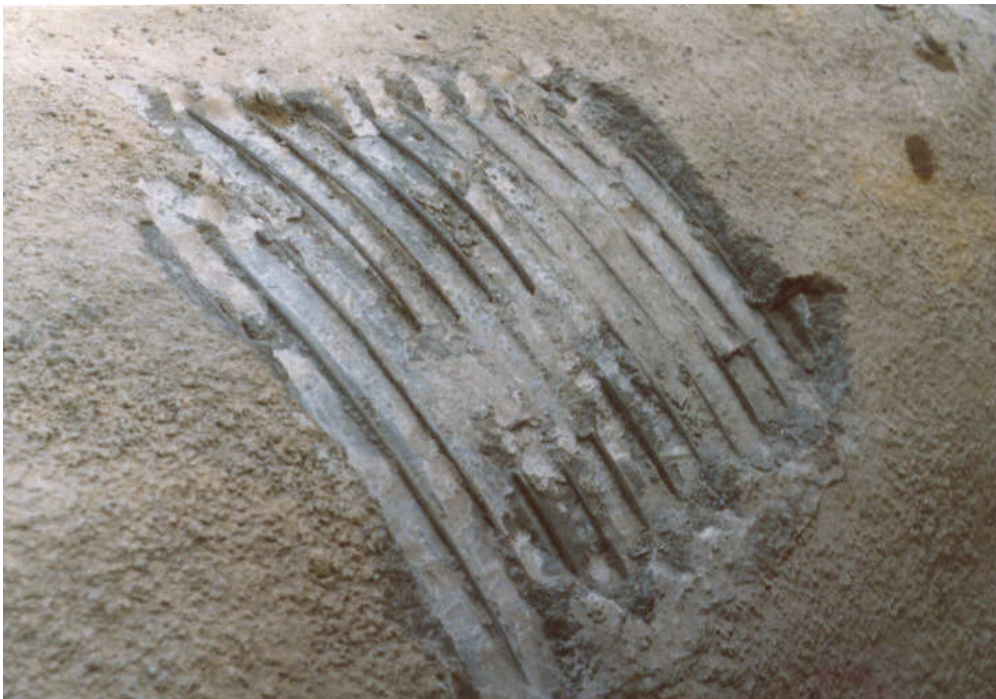
Photograph 1: View of exposed and corroded prestressing wire
