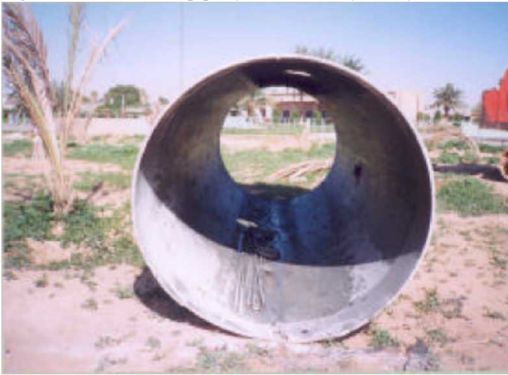
Figure 4 DN1800 GRP pipe after almost 25 years of service
