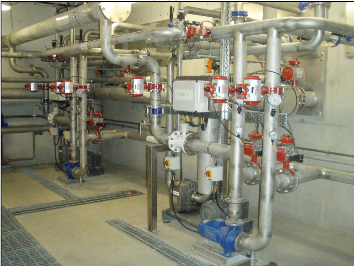
Figure 10 – Membrane Filtration Plant Pump & pipe Gallery (Below Ground)
