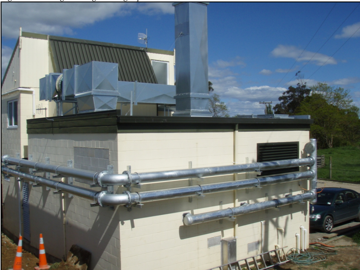
Figure 7- Existing Building Housing Aquamat Process Air Blowers
