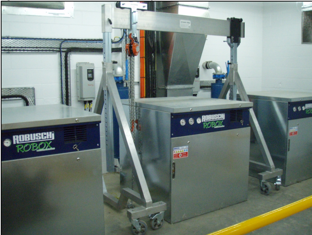
Figure 8- Process Air Blowers Associated with Aquamats
