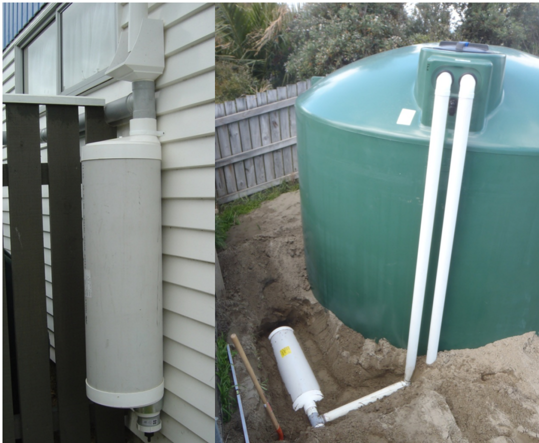
Photograph 2: Buried first flush diverter vs wall mounted unit
