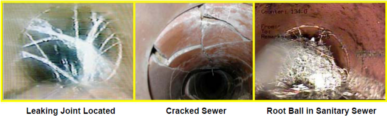
Figure 2: Common sewer faults contributing to infiltration (Colvin, 2004)
