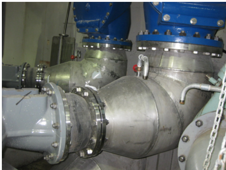
Photograph 5: Discharge Bends off pumps
