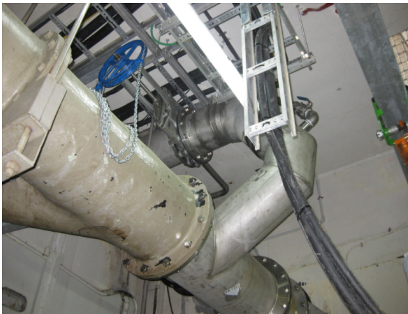
Photograph 7: Cross connection between rising mains
