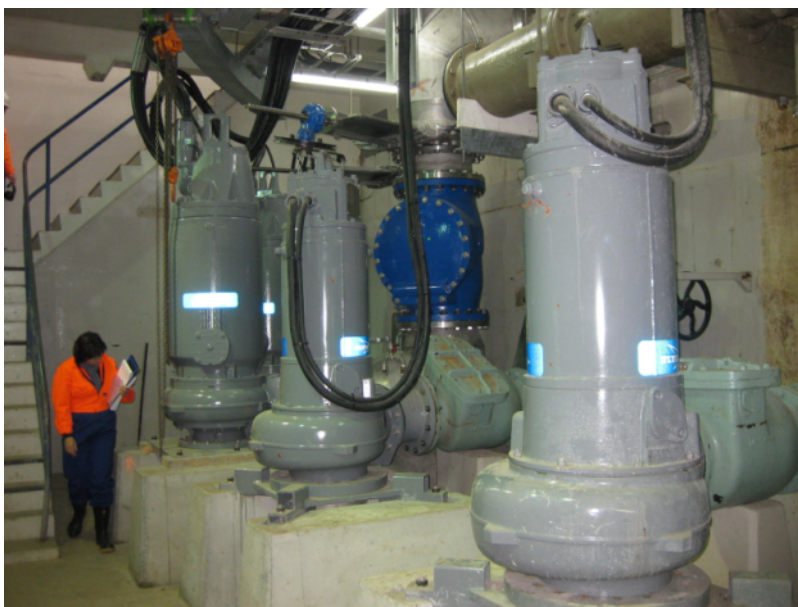
Photograph 8: New installed pumps
