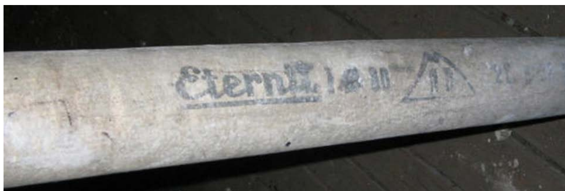
B3-2: Eternit wastewater pipe, installed in an above ground application.
