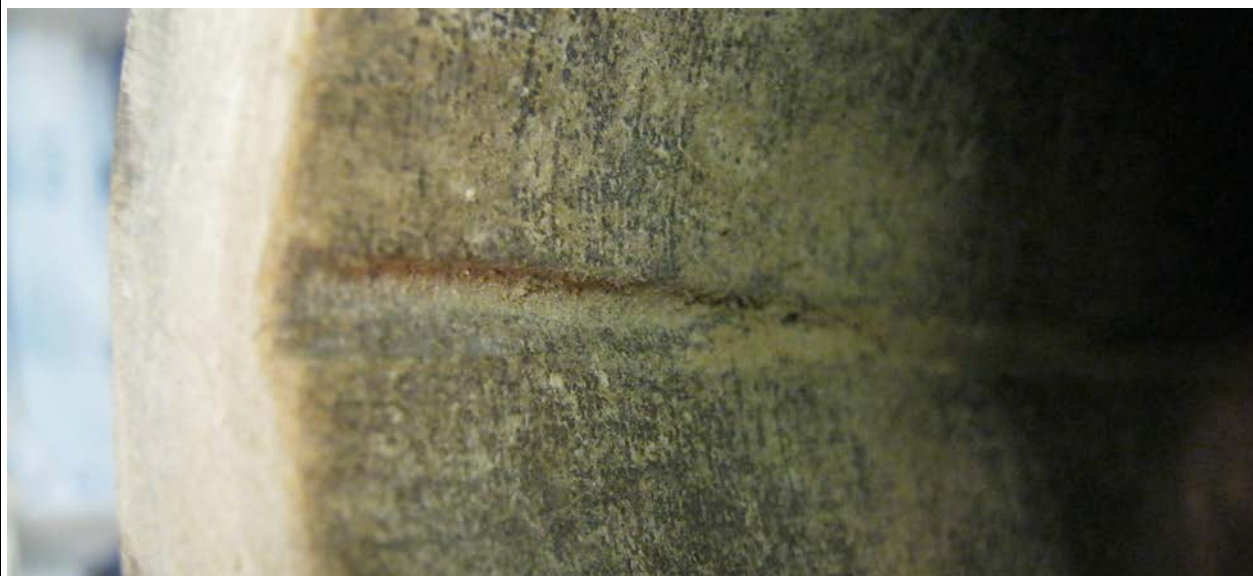
B1-2: Internal view of an Everite pipe, the bitumen lining is still visible. The longitudinal seam from the mandrel joint is clearly visible.
